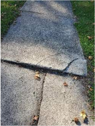
Fair : Uneven and distressed surface that hinders mobility of the average pedestrian. The sidewalk contains surface cracks, vegetation overgrowth, or debris.
