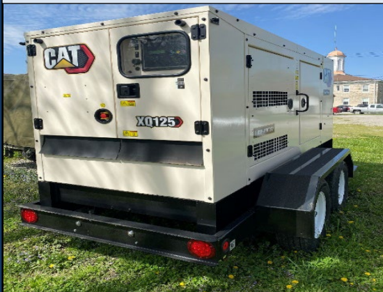
Mobile Generator located at the Ralls County Courthouse in New London, MO
