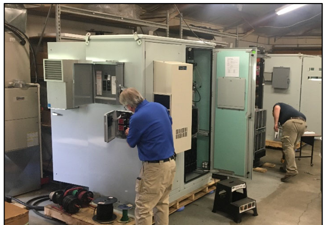
David Serman and Kevin Hall work preparing and programming base radios for a new MOSWIN site.
