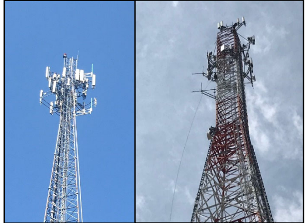
Examples of typical antenna installations at MOSWIN tower
