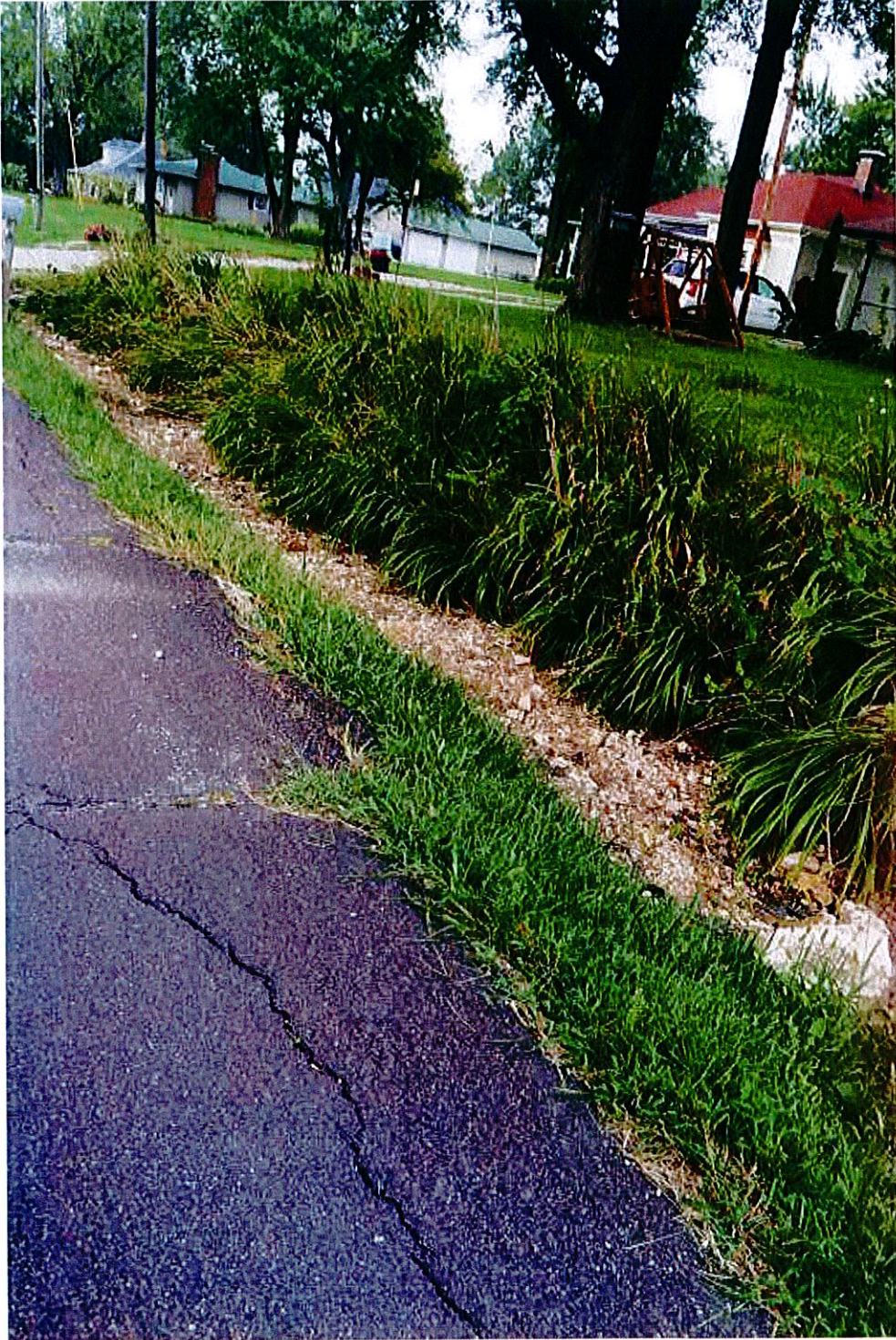
Main St. interrupted ditch
