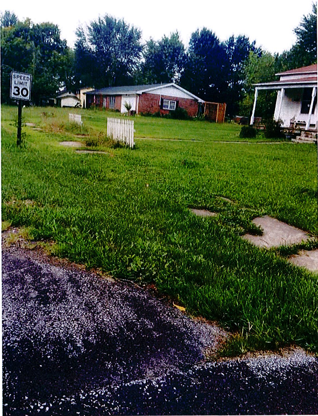
Main St. broken sidewalk
